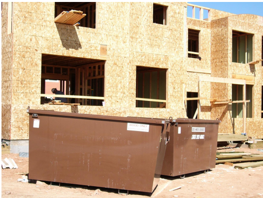
Construction recycling bins are arranged at the site in a manner most conducive to effective recycling efforts
