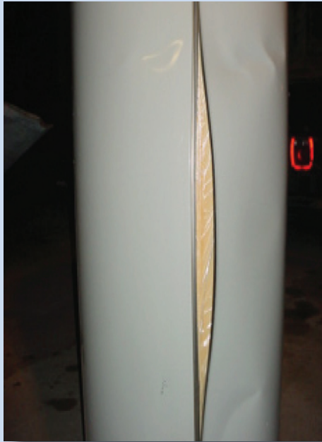
Side splits from a faulty relief valve can cause serious problems in your home.
